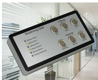
Individual room control panels
