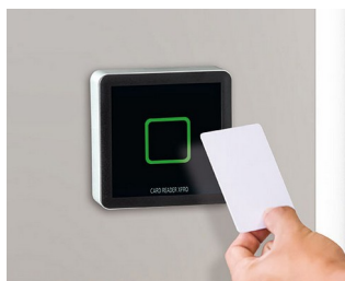
Access control system
