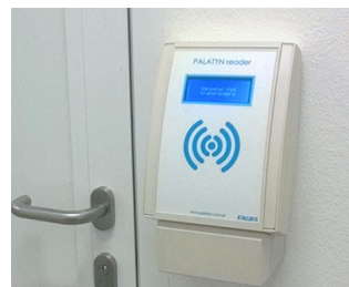
RFID access control readers
