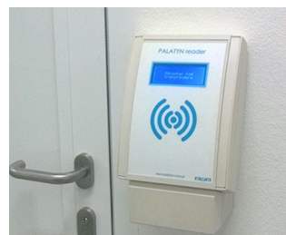
RFID access control readers
