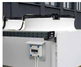
Heating/air conditioning/ventilation control
