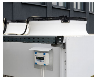
Heating/air conditioning/ventilation control
