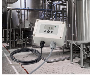
Monitoring with temperature sensor
