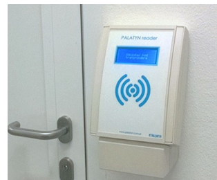
RFID access control readers
