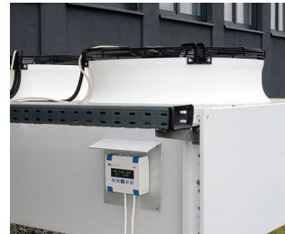
Heating/air conditioning/ventilation control
