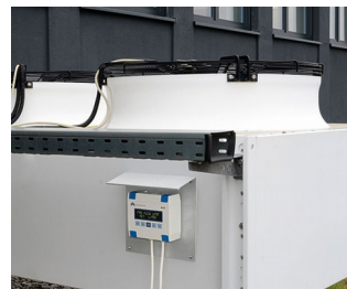
Heating/air conditioning/ventilation control
