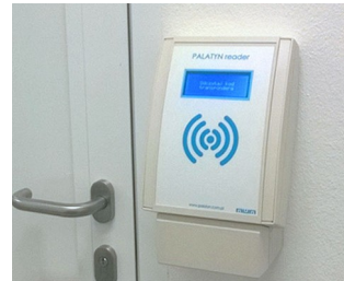
RFID access control readers
