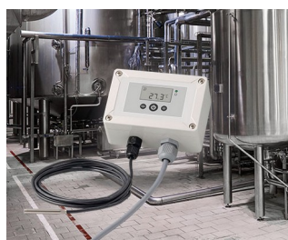
Monitoring with temperature sensor
