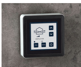
Ventilation system control
