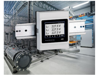
Monitoring of electrical variables
