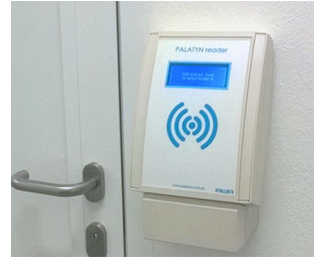
RFID access control readers
