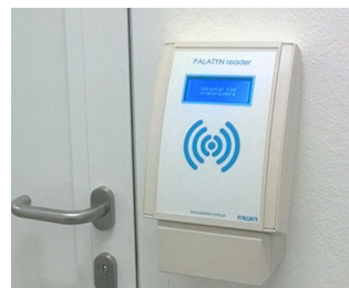
RFID access control readers
