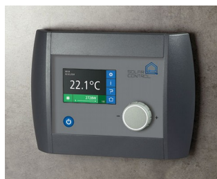
Solar Control Panel
