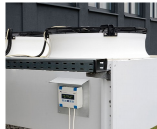
Heating/air conditioning/ventilation control
