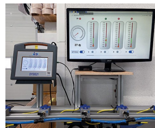
Monitoring system for cleaning nozzles
