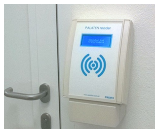
RFID access control readers
