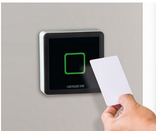
Access control system
