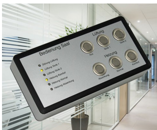
Individual room control panels
