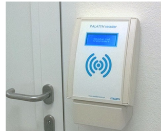
RFID access control readers
