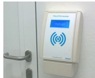
RFID access control readers
