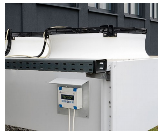
Heating/air conditioning/ventilation control
